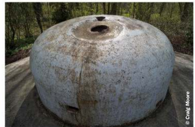
This armoured observation dome was destroyed by the German attack force detonating a shaped charge on top
